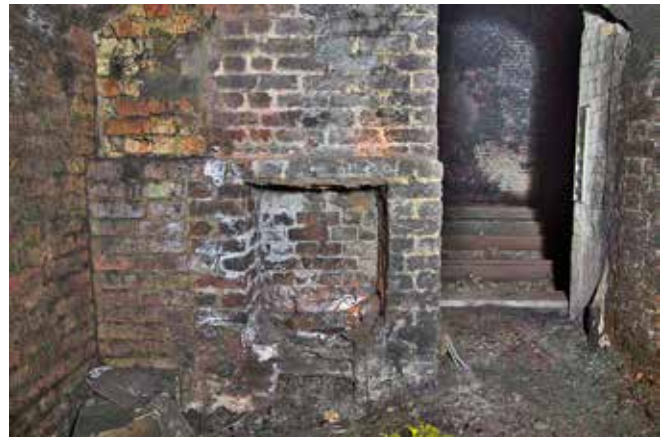
Interior of a crew room inside the tunnel. The chimney from the grate directed smoke into the main tunnel
